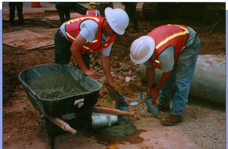
Texas DOT geotechs performed soils investigation and inspection chores. Slump test confirms mix. Cylinders will provide further confirmation of 3,600 psi concrete.
